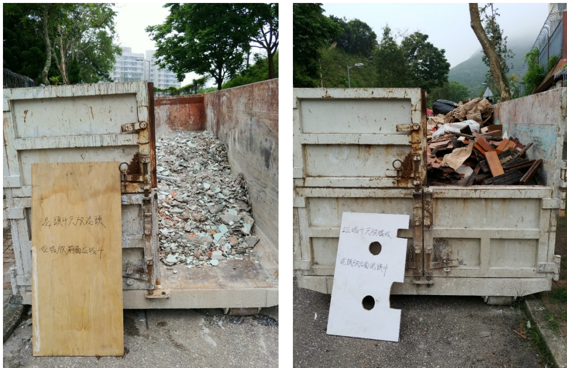
Figure 5.7 Site visit at Site F – Two Separate Dumping Skips for Inert and Non-Inert Waste Storage
